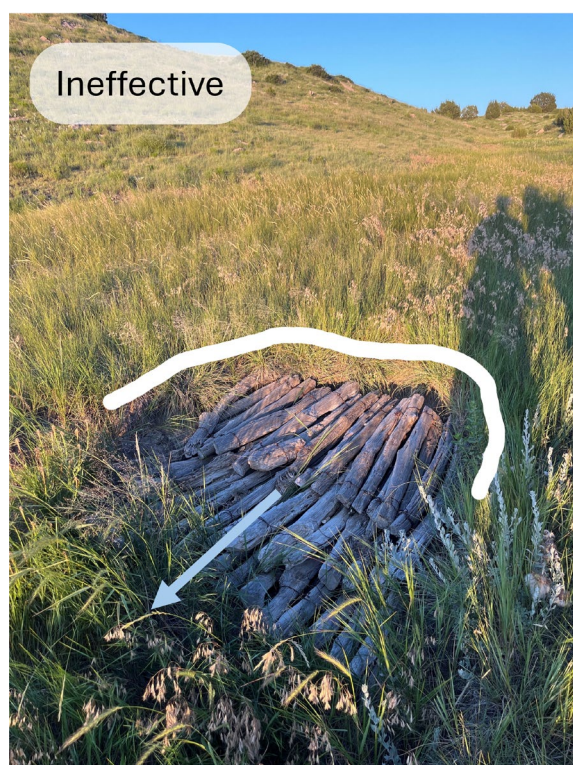
FIGURE 6 | Ineffective log step-fall structure. White outline indicates approximate piping-collapse headcut scarp; blue arrow indicates flow direction. [Color figure can be viewed at wileyonlinelibrary.com ]
